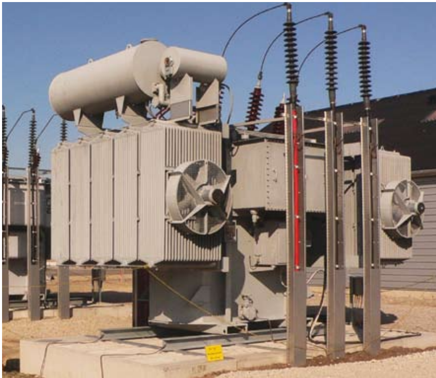
Nordstrand 50/10 kV Transformestation, SEAS-NVE
